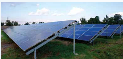
Solar Energy Panels, in HO Alrode
